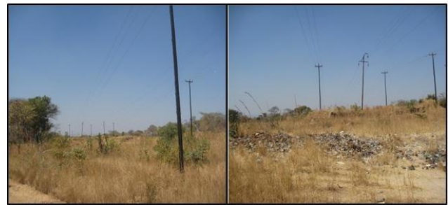
Plate 1: Electricity power lines running across the dumpsite
