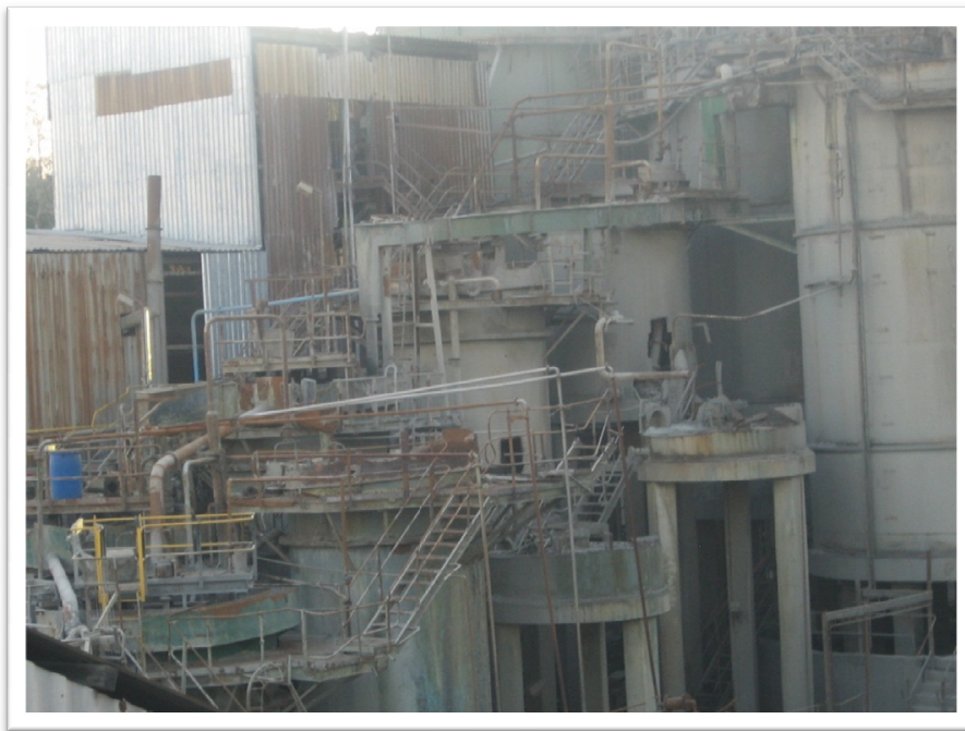
Plate 2: Renco Mine plant with naked electrical wires which might catch fire.
