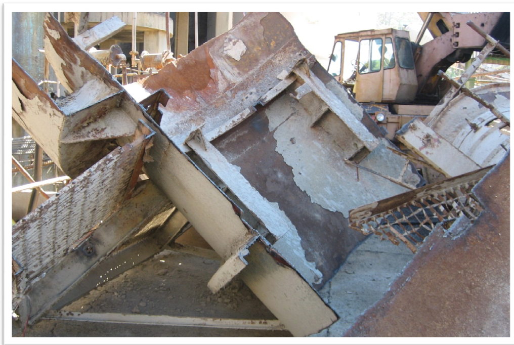
Plate 4: Some section of the plant area where boiler makers were carrying out maintenance work.
