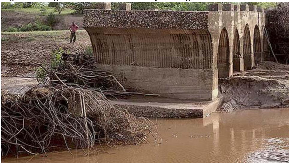
Fig 4 showing the remnants of the Hoya Bridge in Muzarabani.
