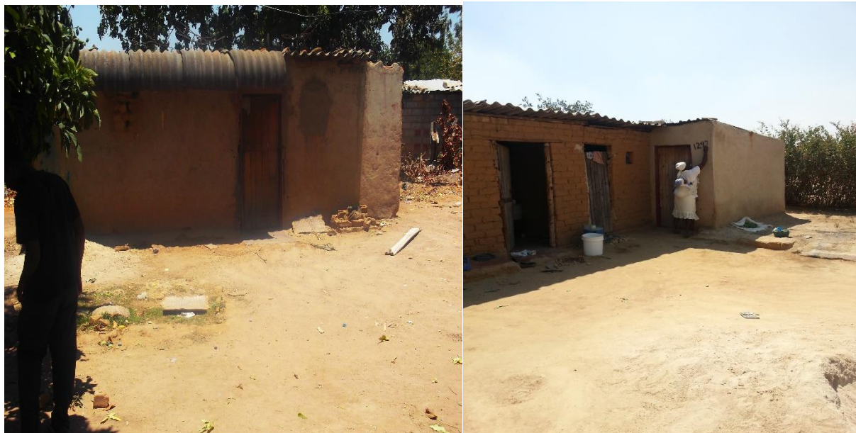
Plate 4. 3 Poorly built houses with green bricks in Epworth ward six.
