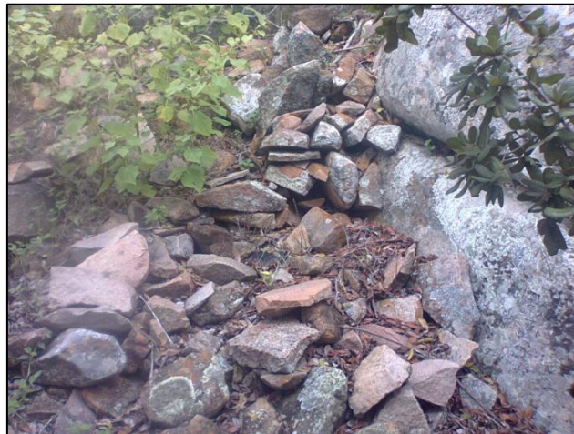
Photo 1 Part of the collapsed eastern walls
