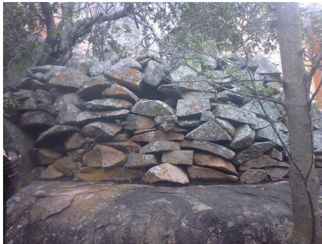
Photo 5 Part of northern wall 1 showing a void
