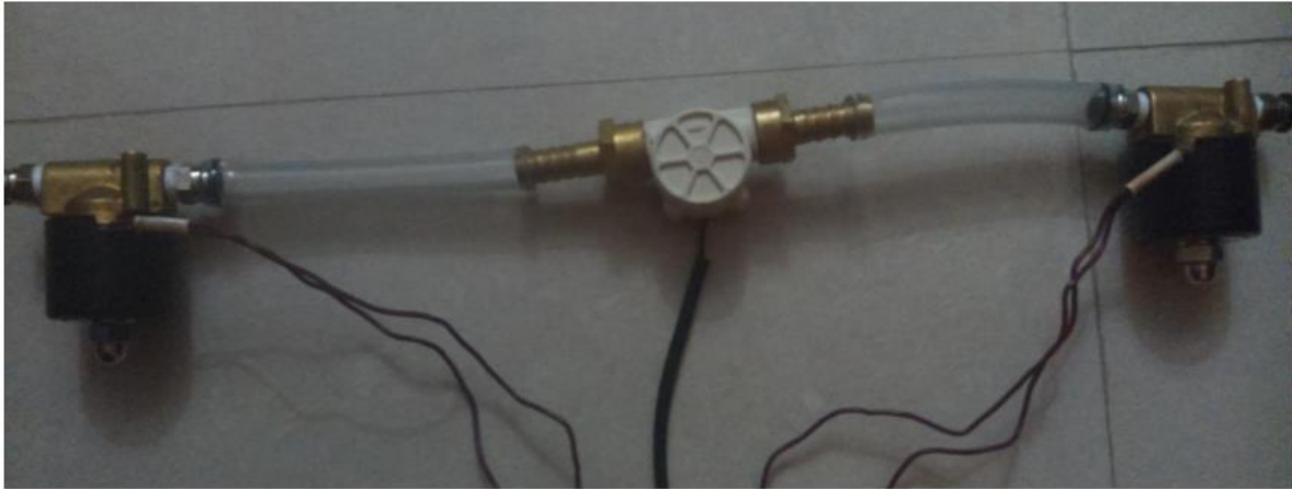
Fig 4.5: Shows water distribution pipe with valves and flow rate sensor.
